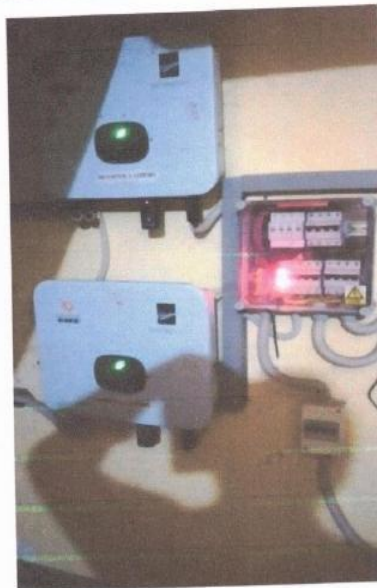
Solar panel photo and inverters
